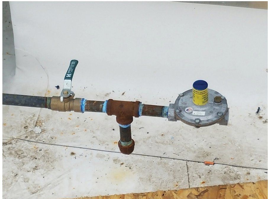
Abandoned natural gas connection.
