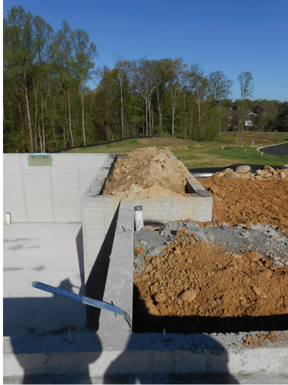
Concrete stem walls supporting more than 4 feet of backfill must have a slab bracing the base of the wall.
