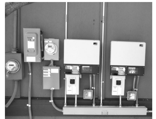
Figure 6: Example String Inverter
