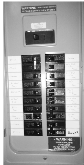
Figure 10: Back-fed Breaker Location
