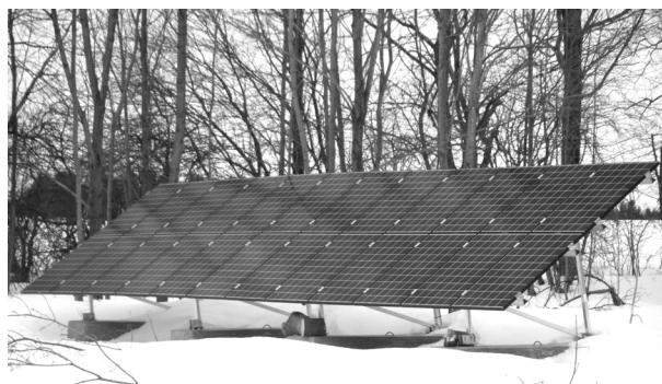
Figure 2: Example Groundmount PV
