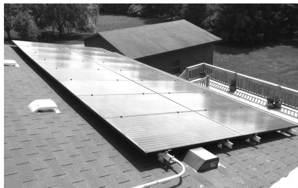
Figure 1: Example Rooftop PV
