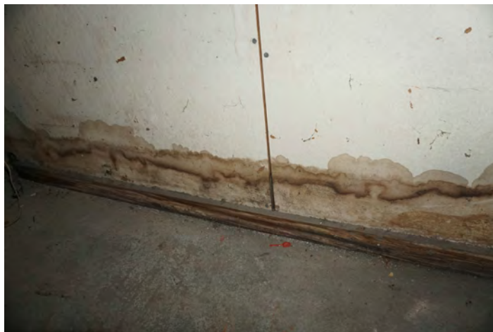
Water Line Inside Building
