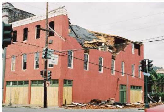
FIGURE 3-7 This vacant building needs significant repair or it will be demolished. (Courtesy of New Orleans [LA] Fire Department)
