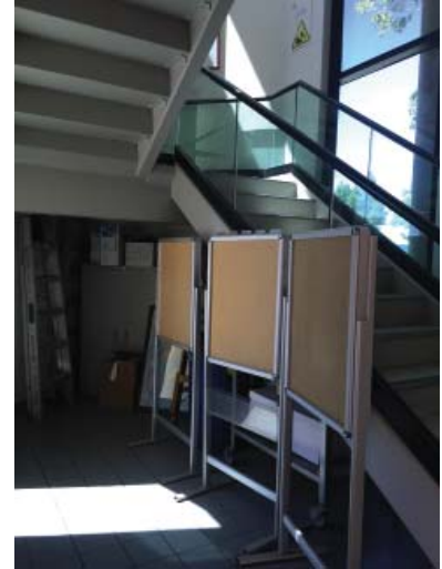
FIGURE 3-1 Ignition of combustible materials beneath the egress stairs can eliminate the stairs as an escape path, and therefore storage in that location is a violation of the IFC.
