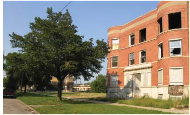
FIGURE 3-8 A vacant building that is not properly safeguarded.
