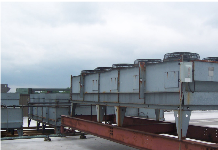
FIGURE 3-9 Condensing unit on rooftop.
